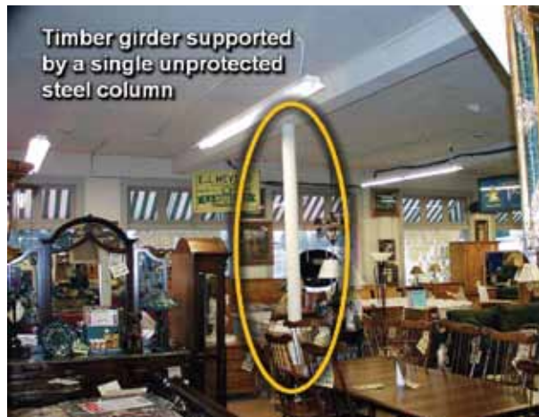
Load bearing masonry wall replaced by unprotected steel columns
